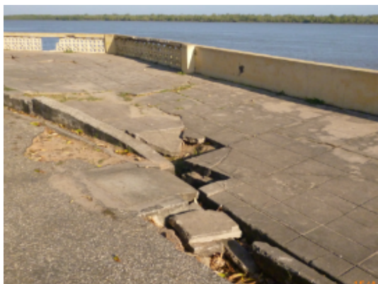
Settlements behind bank wall induced by coastal erosion
