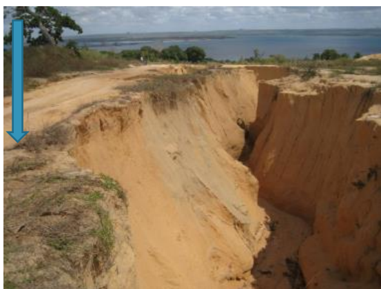
V-shaped erosion gullies throughout Nacala
