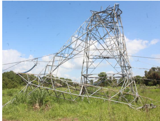
Damage to electric power tower in Mocuba
