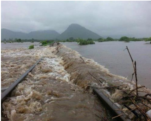
Damage to railways
