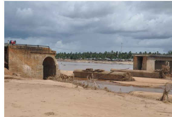
Bridge destroyed on the Licungo River in Mocuba
