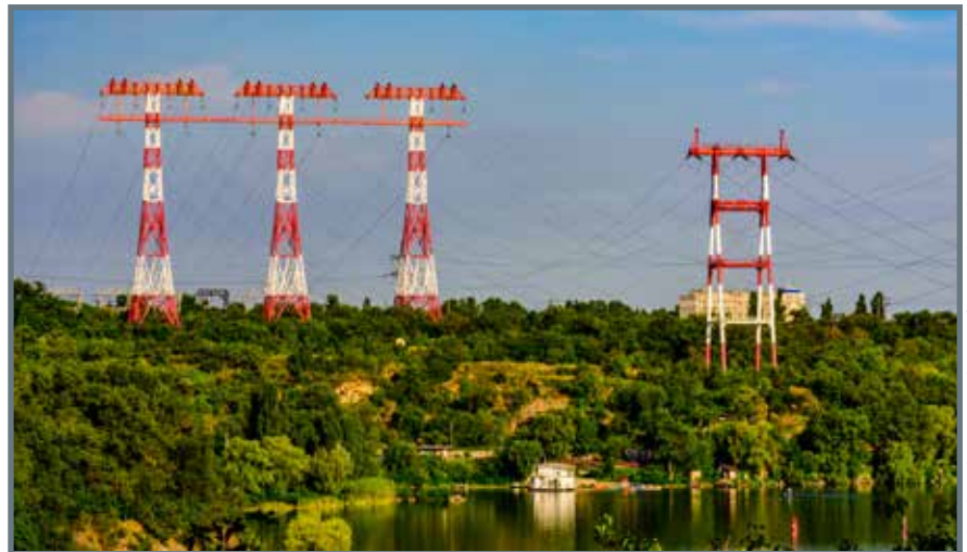
High-voltage lines across the city of Zaporozhye, Ukraine. Photo: Shutterstock.
