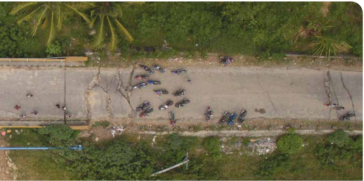
Jono Oge, Indonesia—Collapsed bridge after the September 2018 earthquake and tsunami that hit Central Sulawesi. Photo: Nurwijaya Hariadi.
