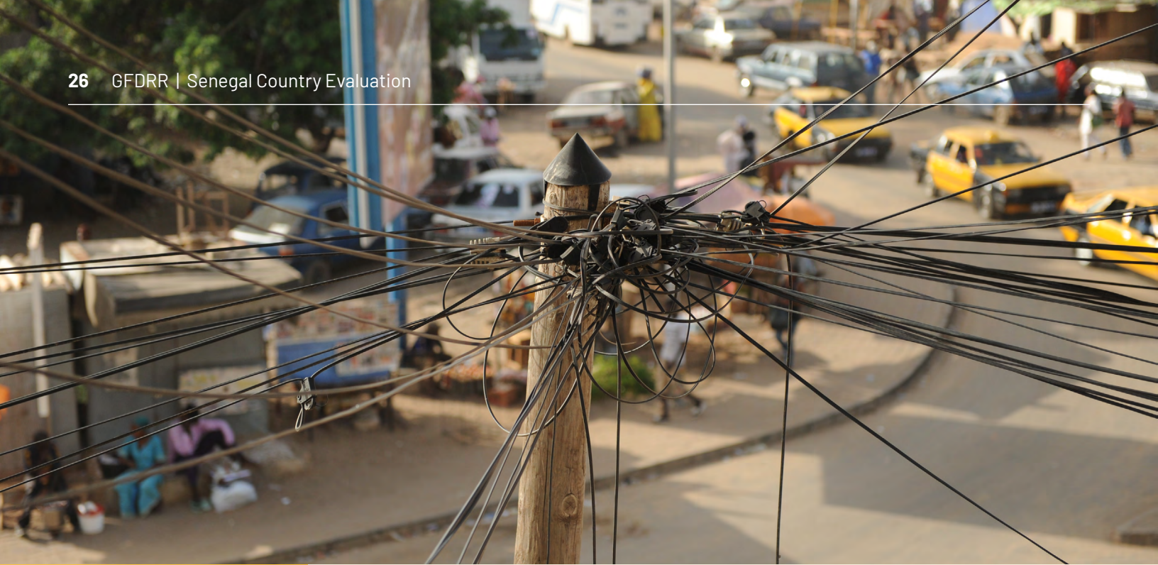
Electric cables in Senegal. Photo: Clement Tardif.
