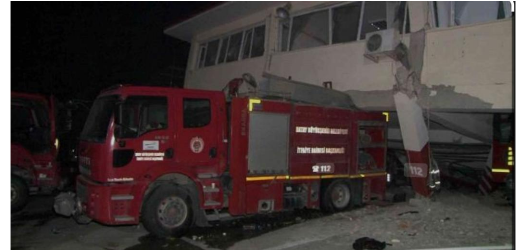
Collapsed firestation during 2023 EQ, Hatay, Türkiye
