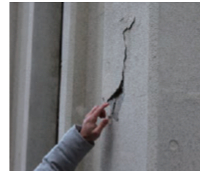
Flaking of mortar
