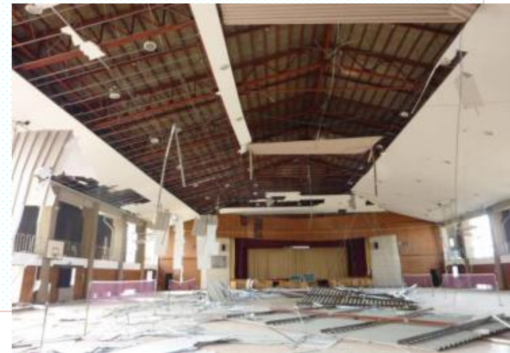
The gymnasium's ceiling collapsed
