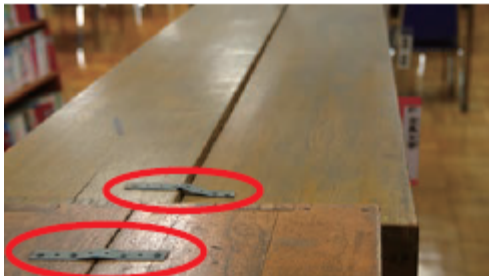
Example where racks are combined and attached together.
