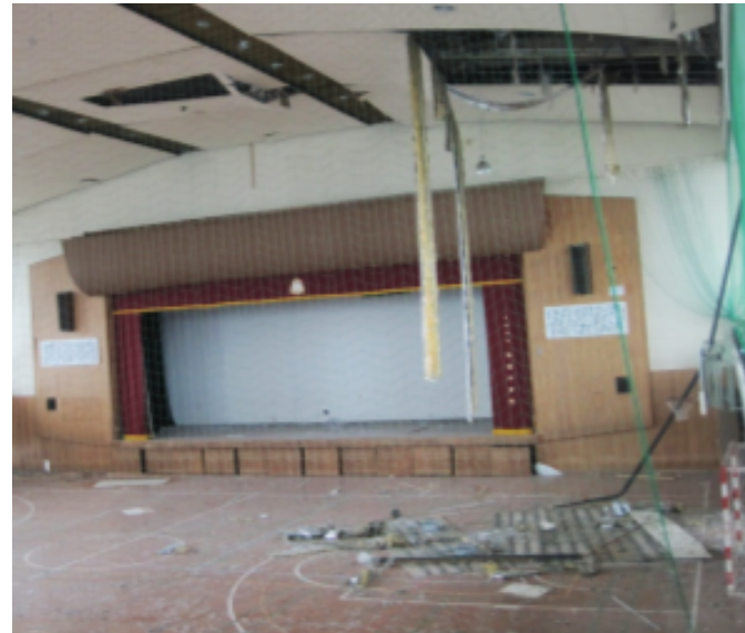
The gymnasium's ceiling collapsed
