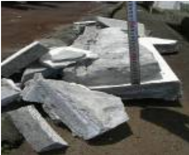
External wall's mortar fell down due to aging
