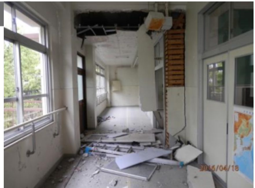
The corridor's ceiling collapsed
