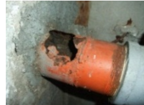
Pipe is broken due to deterioration
