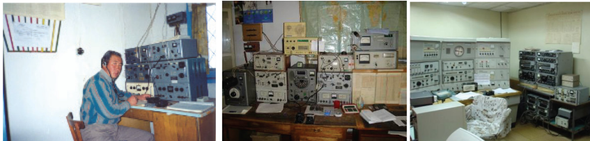
Figure 2.4. Current communication and data transmission equipment at meteorological station (photo 1 and 2 – Kyrgyz Republic), and Message Switching Center (photo 3 – Central Office of Turkmenhydromet).
