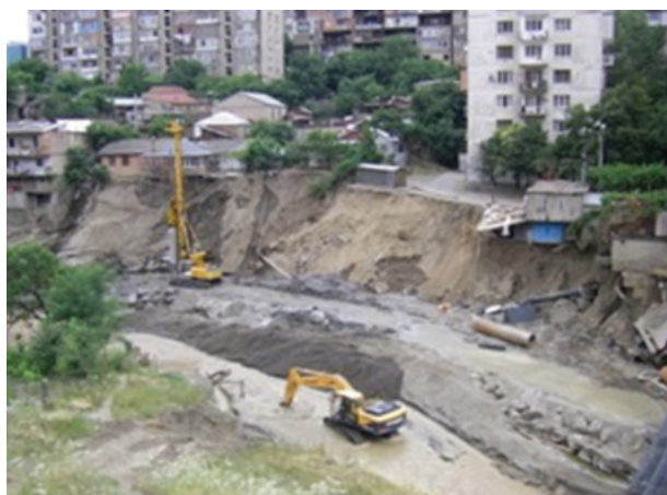
Figure 5: Eroded riverbank downstream from Vere River tunnel no. 1
