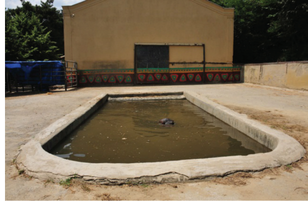
Figure 16. Damaged Animal Enclosures
