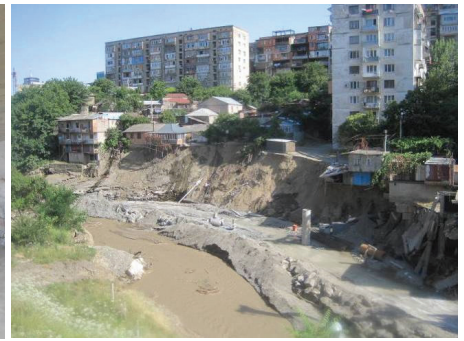
Photo 3.7 Flood Scoured RB of Vere River d/s from Tunnel 6 showing undermining of Buildings
