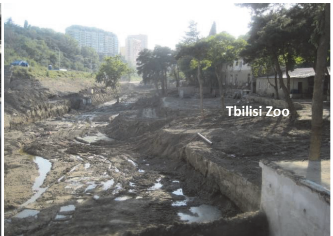
Photo: 3-15 looking upstream at same location as Photo 3-14 from the Tbilisi Zoo
