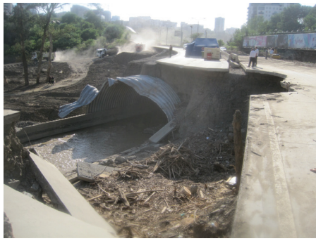
Photo 3.12 Flood Damaged Exit to Tunnel 2
