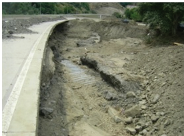
Figure 3: Damage to the Amirejibi Highway close to Vere River tunnel no. 5
