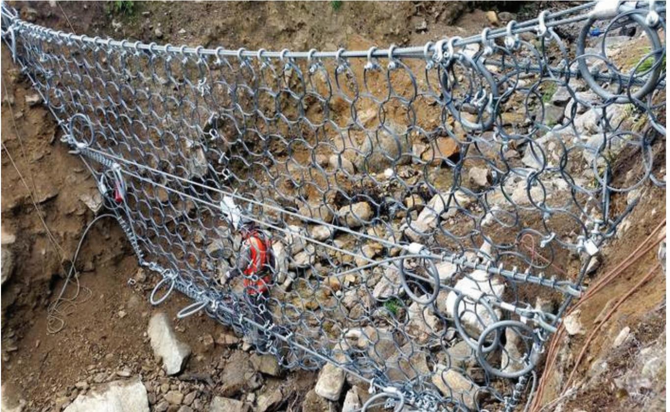
Photo E. 23. Debris flow barrier for secondary watercourses
