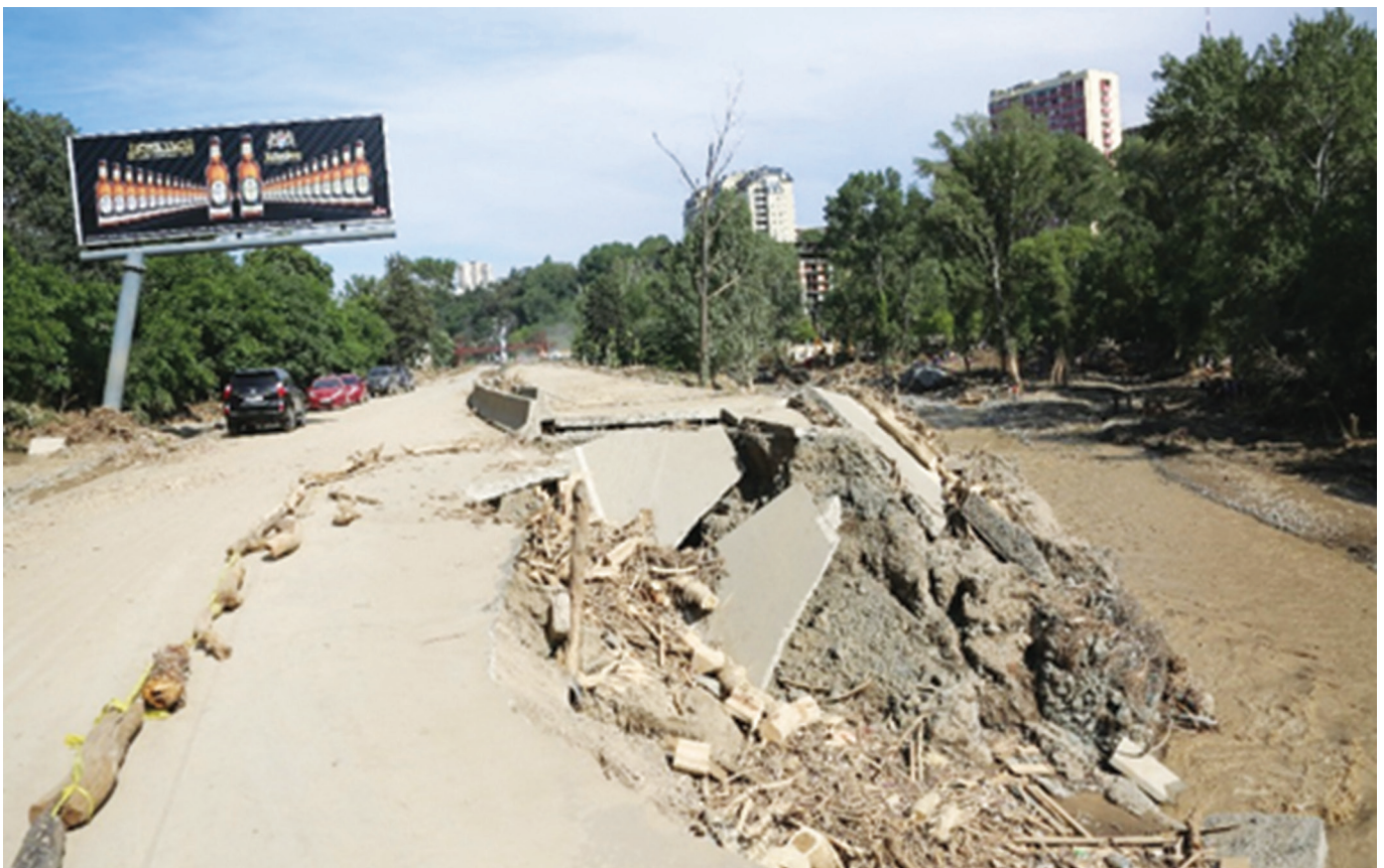
Figure 9: A collapsed section of the Amirejibi Highway.
