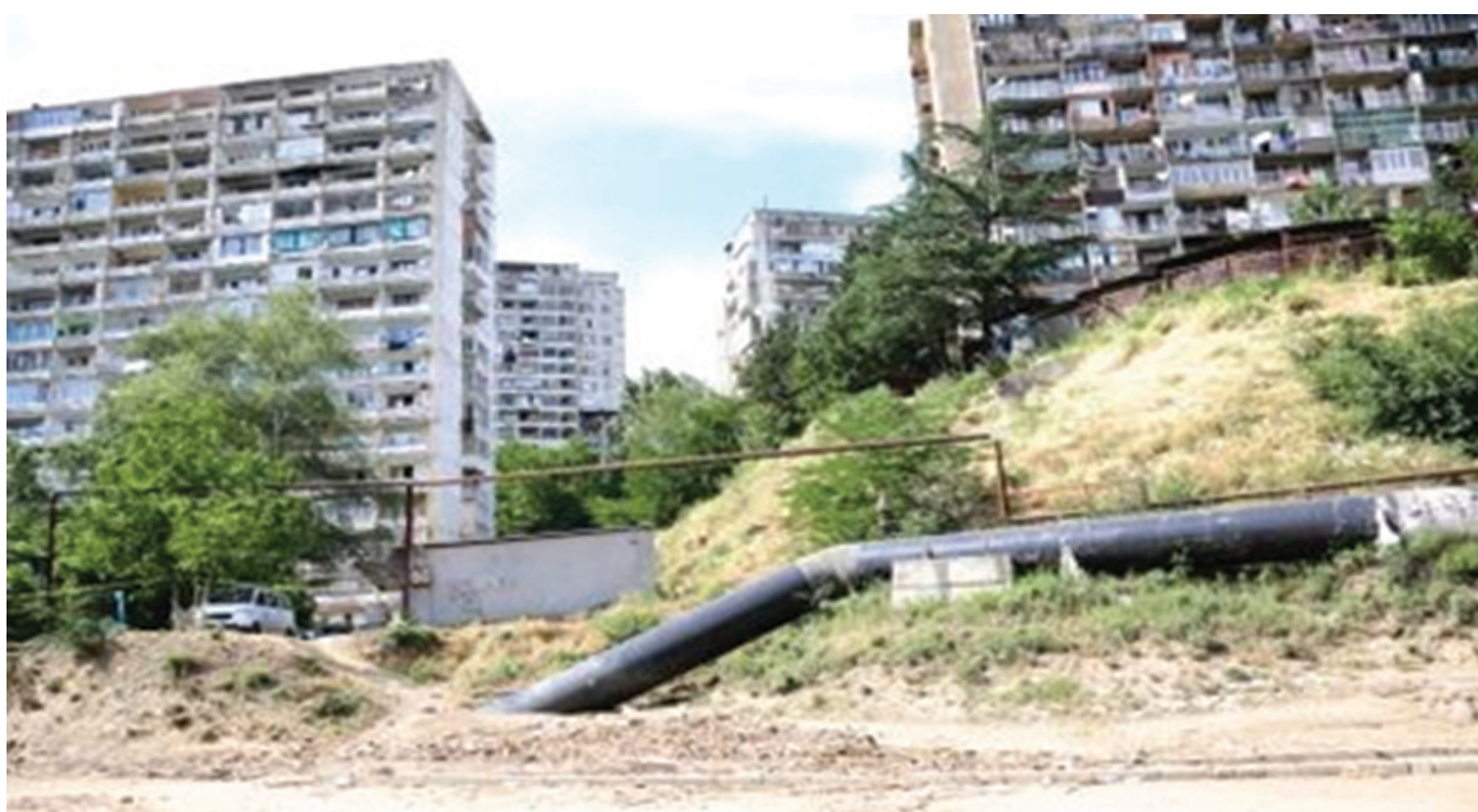
Figure 11. The 800 mm. high-pressure main water pipe
