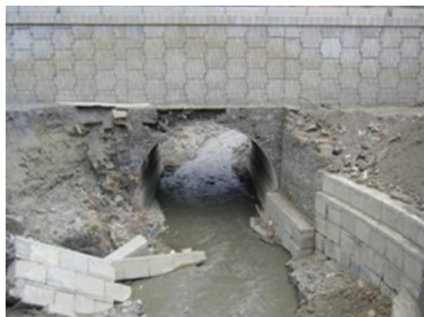
Figure 4: Damage to the gabion and concrete inlet protection walls of Vere River tunnel no. 5
