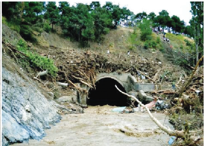
Photo 3.4 Inlet to 1958 Tunnel after Flood
