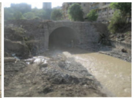
Photo 3.10 Flood Damaged Exit to Tunnel 4
