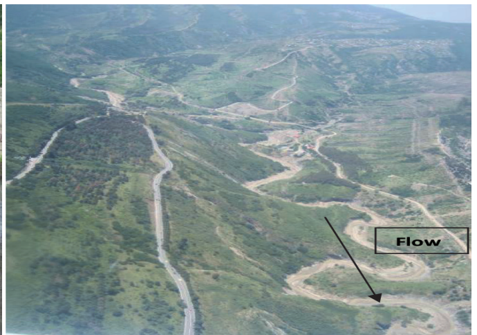
Photo D.6 Proximity of Road to Tskneti to Steep Slopes Close to Vere River
