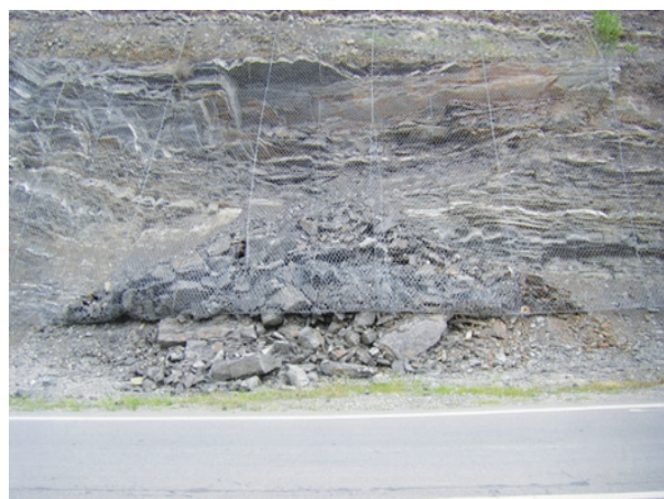
Figure 8: Cut rock slope failure along the Amirejibi Highway. Stronger netting is required.
