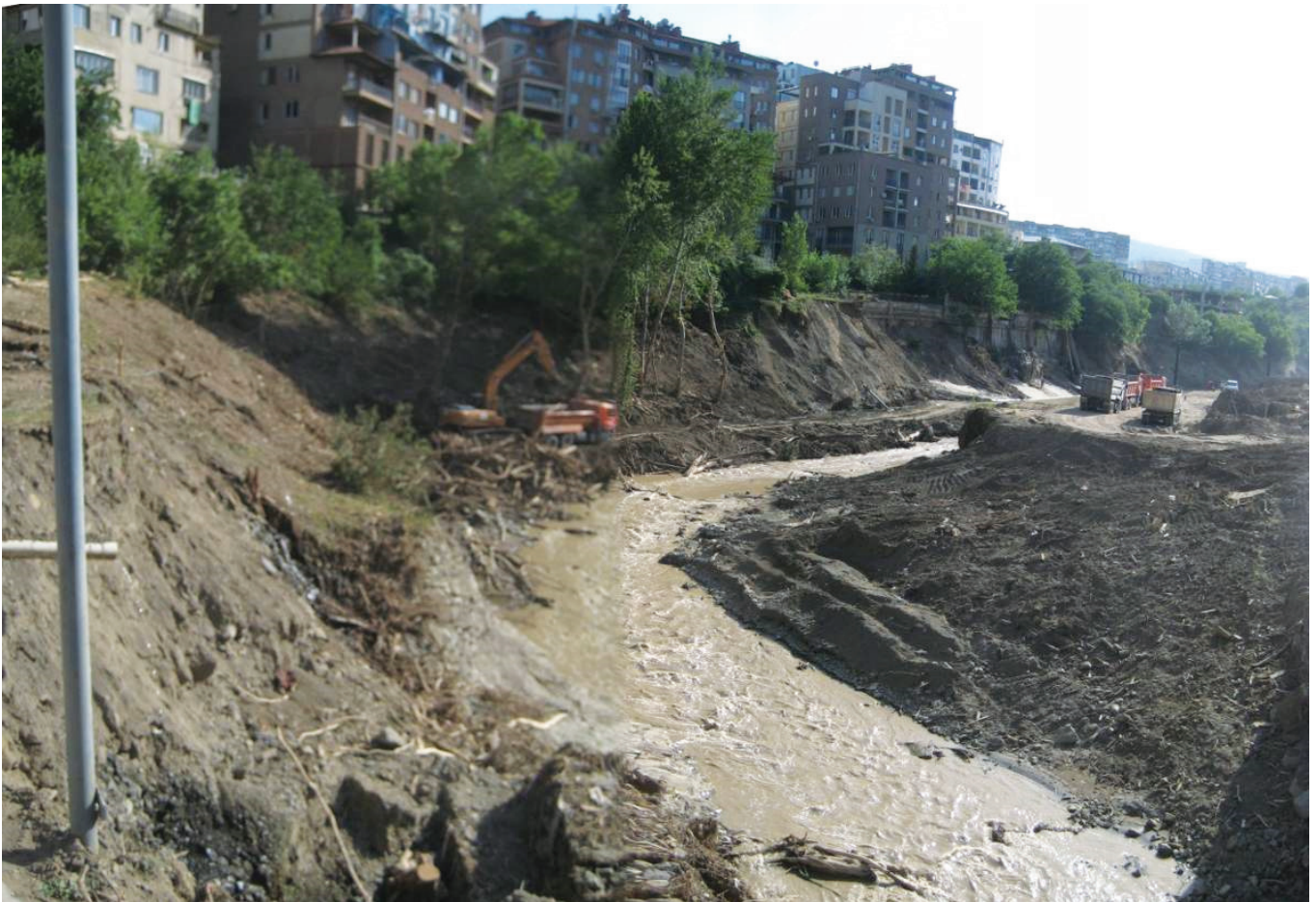
Photo E. 14. Unstable right river bank in this section between Tunnel 6 and 5
