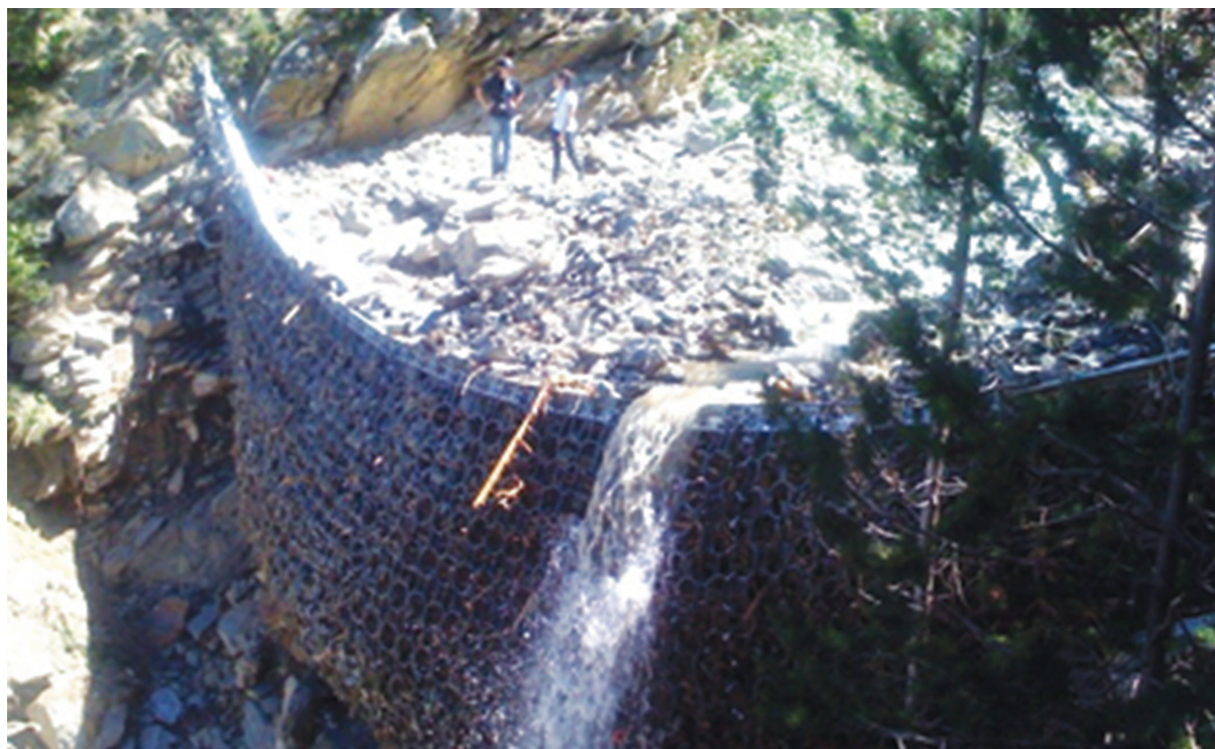
Figure 15: High-capacity debris flow steel nets
