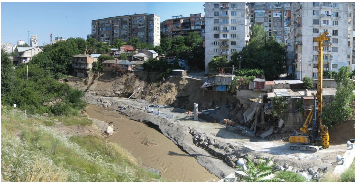
Photo E. 13. Unstable right river bank in this section between Tunnel 6 and 5
