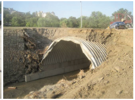
Photo 3.13 Flood Damaged Entrance to Tunnel 1
