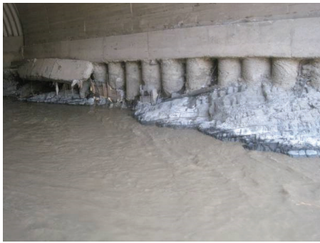
Photo 3.5 Outlet from Tunnel 6 showing extent of Scouring of Bed
