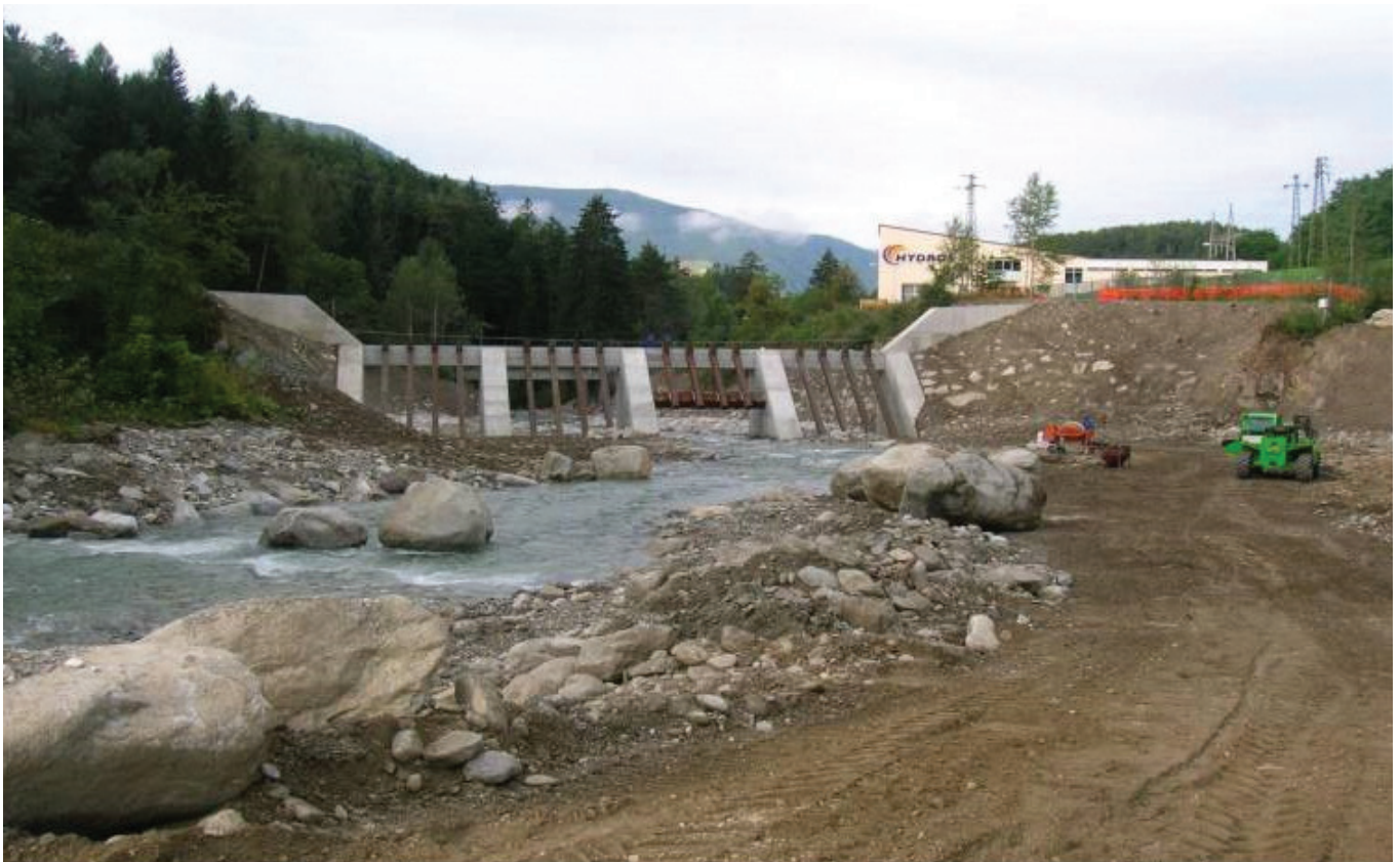
Photo E. 27. Selective Barrier for floating load (debris timber)
