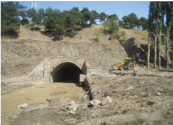
Photo 3.3 Inlet to 1958 Tunnel Cleared After Flood
