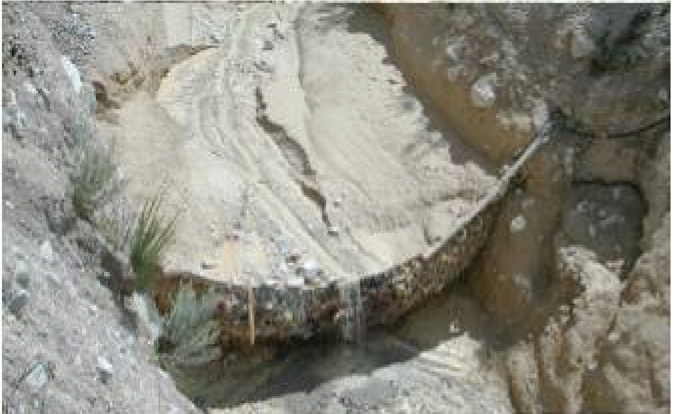
Photo E. 25. Debris flow barrier for secondary watercourses, with debris materials collected, it forms a natural weir
