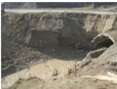
Photo 3.8 Flood Damaged Entrance to Tunnel 5
