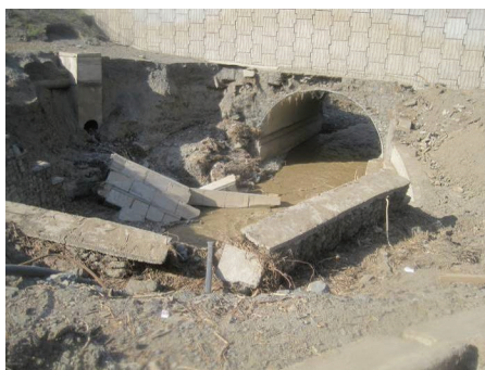
Photo 3.9 Flood Damage to 2nd Part of Tunnel 5
