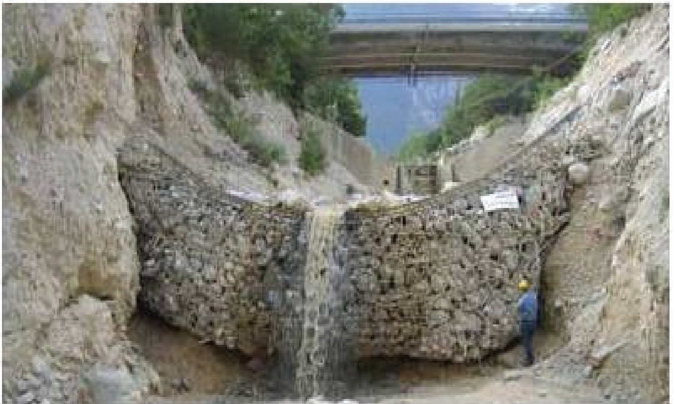
Photo E. 24. Debris flow barrier for secondary watercourses, with debris materials collected, it forms a natural weir
