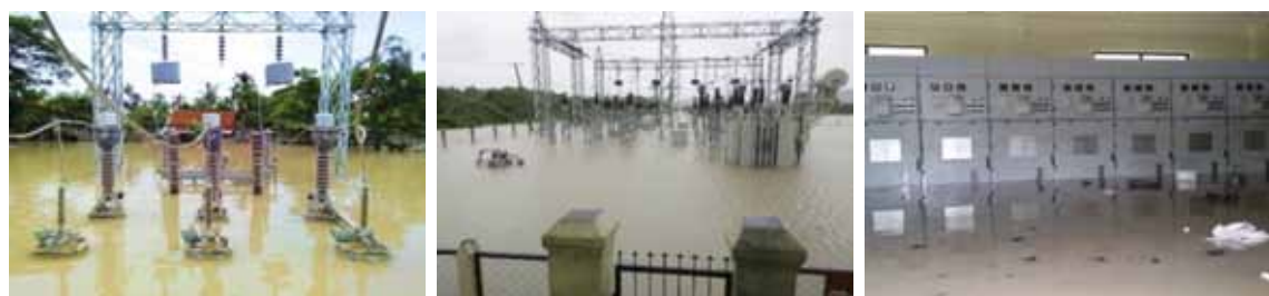
Submerged substations and control rooms in deep water.
