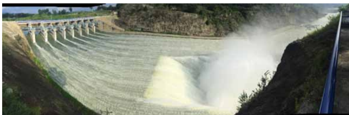
Figure 20. Damage to spillway channel at Kyeoo Kyeewa Dam in Magway Region
