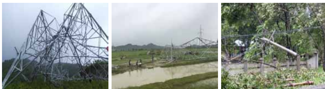
Collapsed towers and poles.
