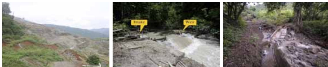
Dams, water canal, and weir damaged by floods.
