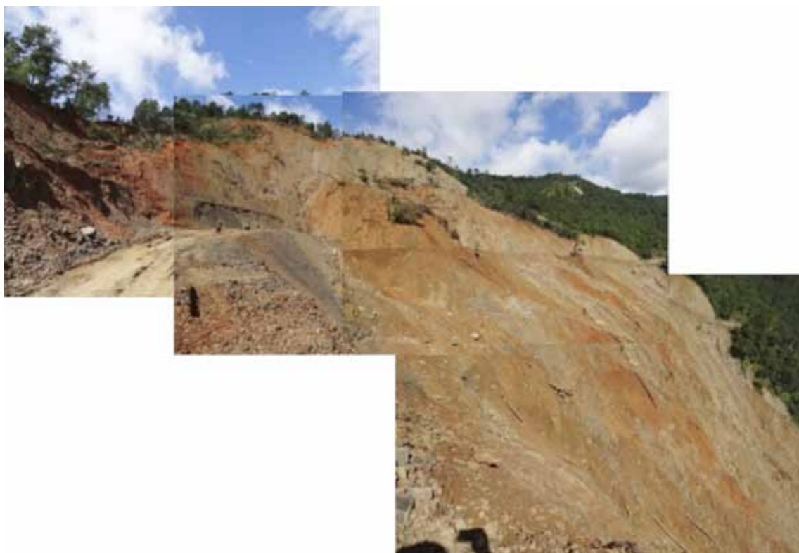
Figure 35. Road formation failure on Kalay-Falam-Hakha road in the Chin State
