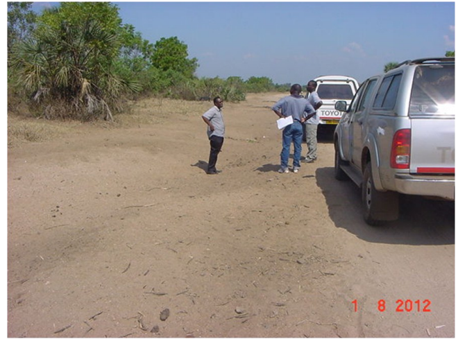
Part of the damage to the road within the Mbwazi AD-MARC and Makhanga Stretch
