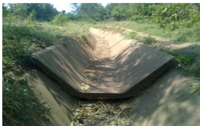
Fig 7: A section of damaged irrigation canal in Muona Irrigation Scheme
