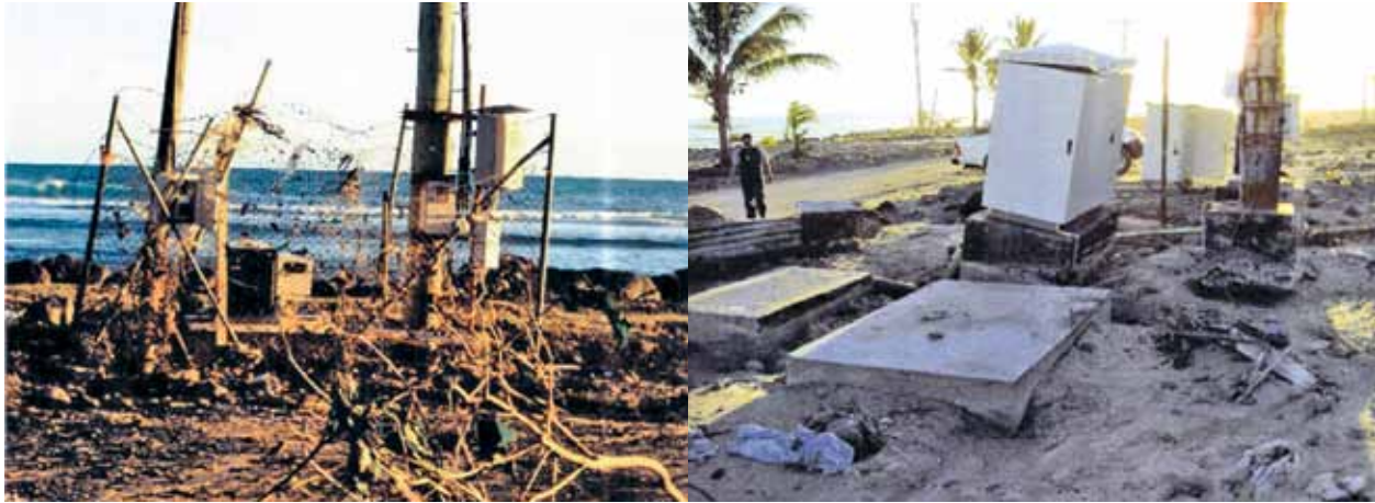
Figure 15. Damaged telecommunications sites
