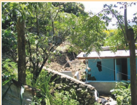
a. Minor landslide where the impact of the debris has damaged a concrete home.
