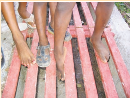
FIGURE 7.33 Some construction practices can pose dangers to small children
