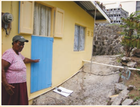
a. Resident indicating maximum observed flood levels prior to intervention.
