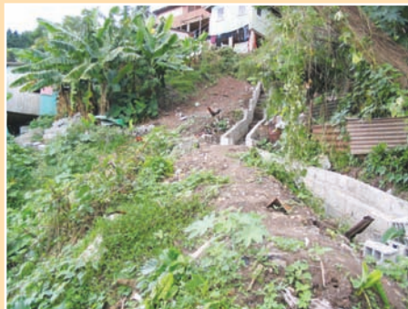
FIGURE 6.9 Drain aligned to intercept surface water and routed around a major preexisting landslide
