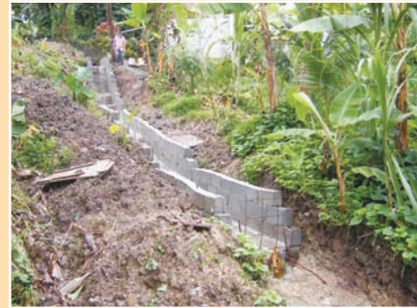
FIGURE 6.18 Poor practice: Downslope drain construction begun at top of hillside rather than base of slope
