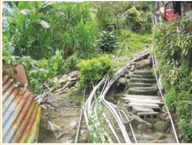
a. Unauthorized housing is often supplied with water delivered through plastic pipes.
