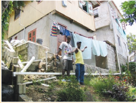
a. Connection of household roof water to a nearby main drain.
