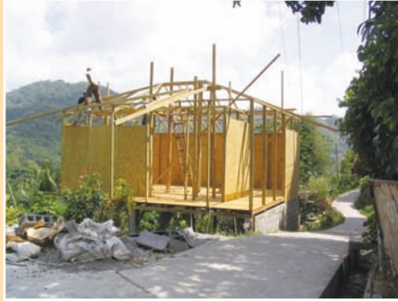
FIGURE 8.16 Absence of building controls can lead to inappropriate construction
