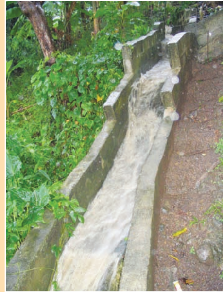
a. Discharge in a stepped drain during a major storm event indicates adequate capacity.
