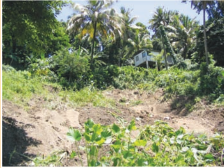
FIGURE 3.8 Postfailure slope stability
