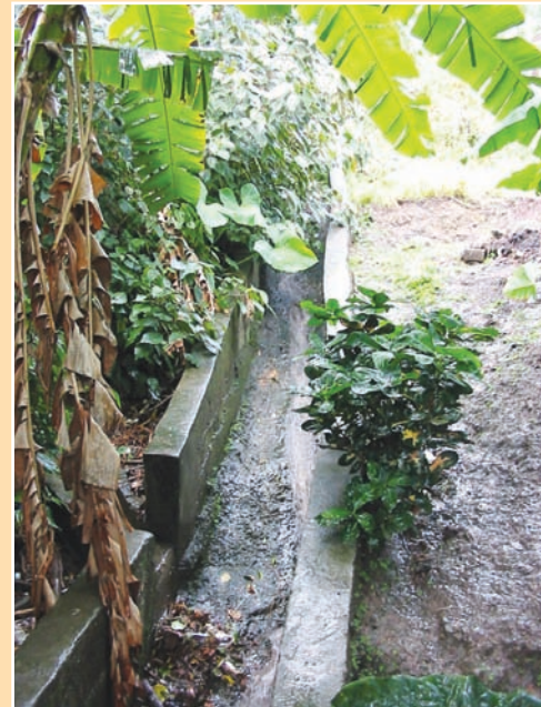
b. A drain built in a natural drainage channel with high side walls prevents surface runoff entry.
