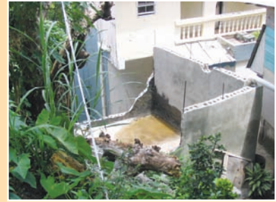
c. A water tank constructed of a single skin of blocks which failed and caused significant downslope damage. Such structures have the potential to trigger slope instability.
