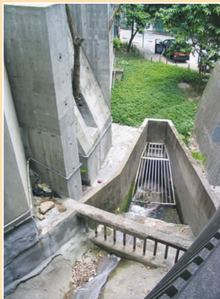
FIGURE 6.23 Debris trap in an urban area of Hong Kong, SAR, China
