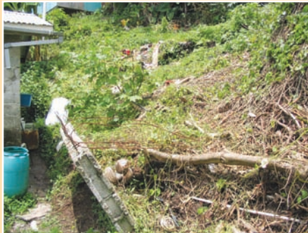
a. Typical failure of modest retaining wall built by resident.
