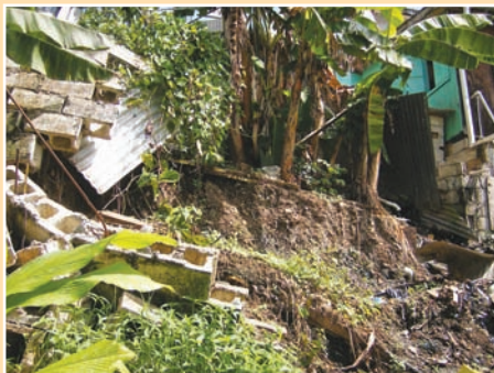
b. Retaining wall built by resident failed, with lower part of wall displaced to rear of property.
