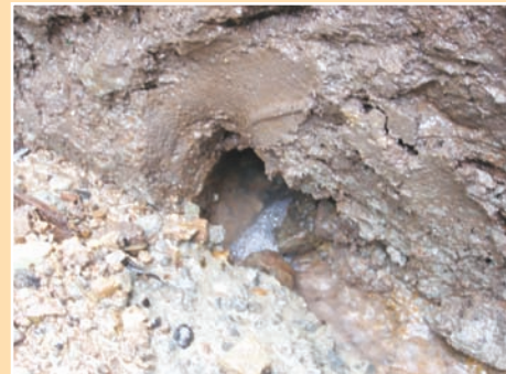
FIGURE 3.21 Exposed soil pipe some 30 cm below the soil surface
