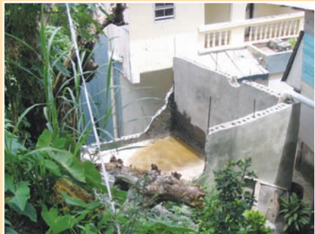
FIGURE 5.15 Potential landslide hazard driver: Failure of poorly designed and constructed water storage structure
