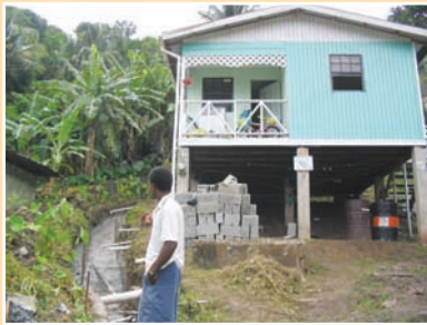
a. Show home located prominently within a community; note gray water pipes connected to a new drain.
