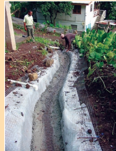
f. Finishing the drain with a cement skim on the drain base.
