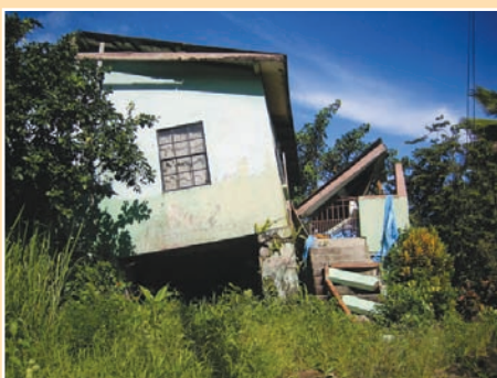
b and c. Worsening of cracks attributable to a progressive landslide which continued to move over a four-year period, finally resulted in a complete loss of property.
