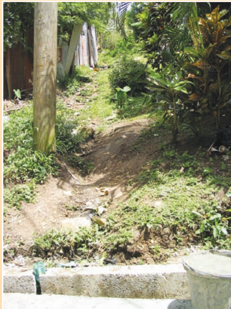
a. An eroded earth footpath also acts as a drainage route and causes the lower concrete path to flood.
