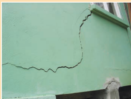
FIGURE 5.17 Cracks in a wall: Past slope instability or poor construction?
