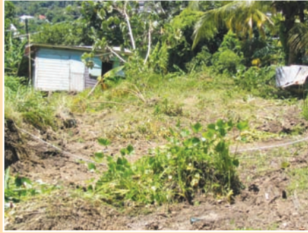
FIGURE 5.16 Evidence of minor slope movement
