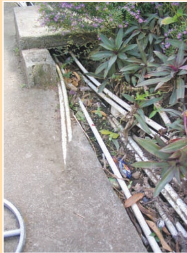
e. Small footpath drain rendered completely ineffective by routing water supply pipes along its length.
