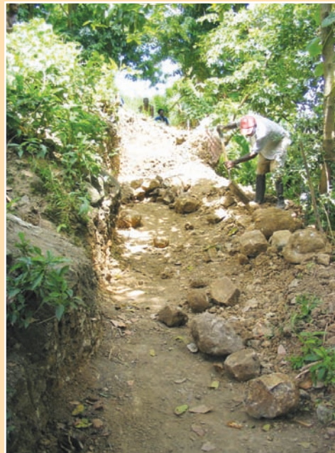
b. This intercept drain, when completed, was regularly used by criminal groups for rapid access to and escape from adjoining properties.
