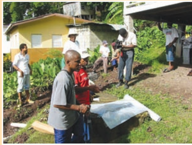
a. Community leaders, residents, local contractors, and site supervisors assemble on site to begin construction of a low-cost drain.
