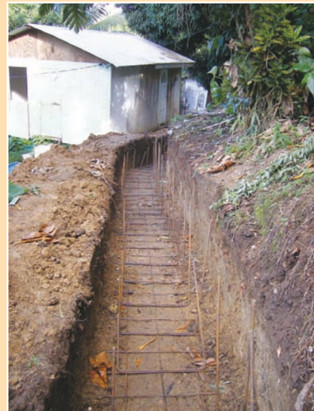
FIGURE 7.17 Example of detailed alignment issue encountered at construction start
