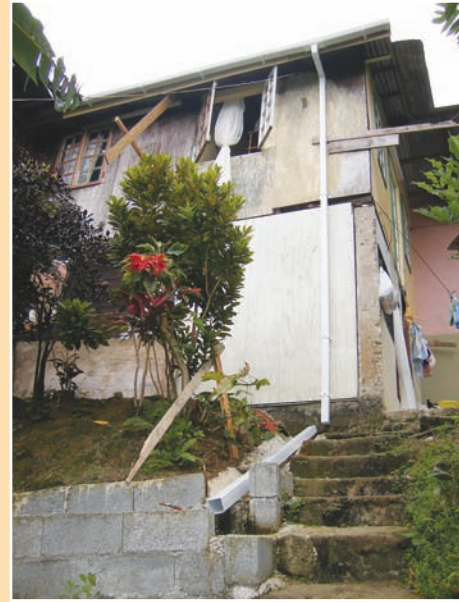
FIGURE 7.6 Connection of downpipe to drain awaits purchase of a connecting section
