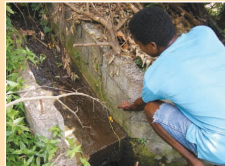
b. Resident notes maximum depth of observed flow in a recently constructed drain during a storm event.
