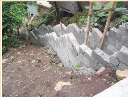
FIGURE 7.31 Drain built with inappropriately high sidewalls
