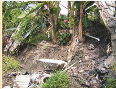
b. Slope failure caused by lack of water management from upslope unauthorized housing.
