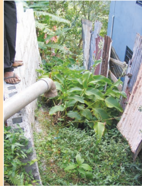
a. Water-demanding plants (dasheen, center) indicate saturated soil near gray water outflow.
