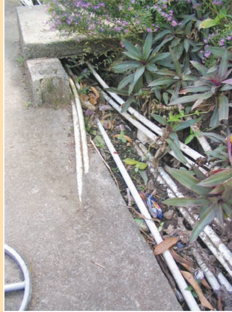
b. Water supply pipes may have been laid in drains for ease of installation, thus reducing drain capacity.
