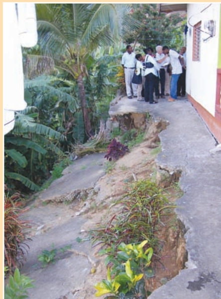
FIGURE 5.13 Potential landslide hazard driver: Cutting platforms to build houses
