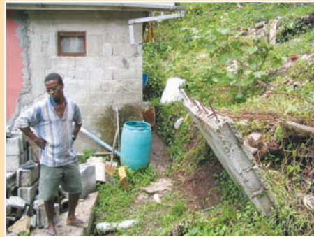
b. Resident in area of slope instability adjacent to his home prior to a MoSSaiC intervention.
