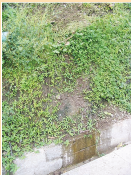
FIGURE 5.11 Seepage occurring in dry weather conditions where there is no sign of a zone of topographic convergence
