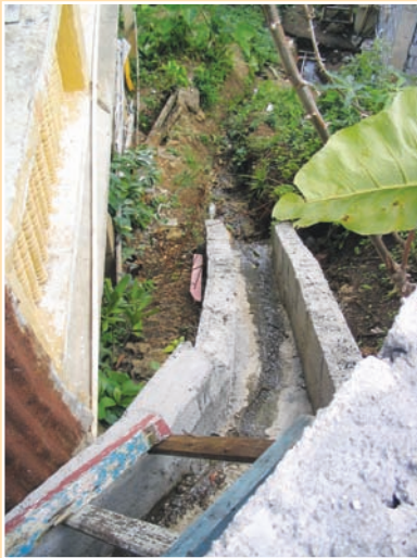
d. A drain that is incomplete and may thereby cause instability downslope.
