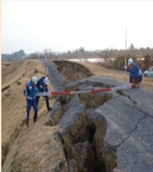
FIGURE 2: Damage to the river dikes at Narusegawa
