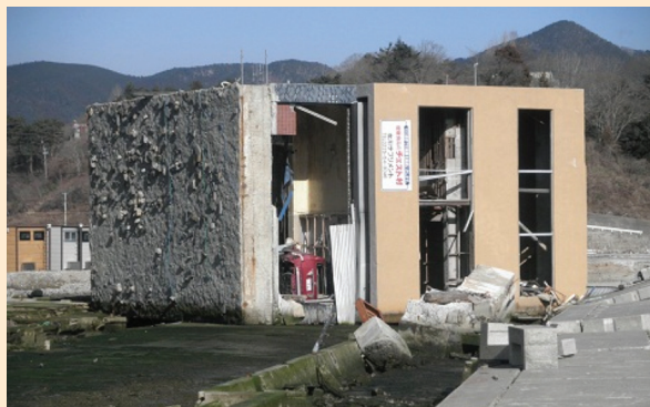
FIGURE 7 (bottom): Overtured building of reinforced concrete with pile foundation
