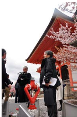
Fire hydrants all around the whole complex
