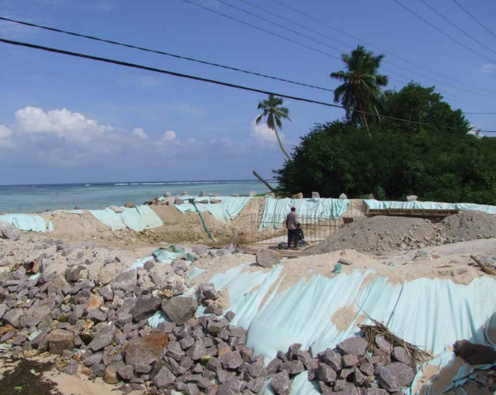
Mahe Island, Seychelles – Works to protect against river mouth sanding and coastal erosion. Photo credit: GFDRR
