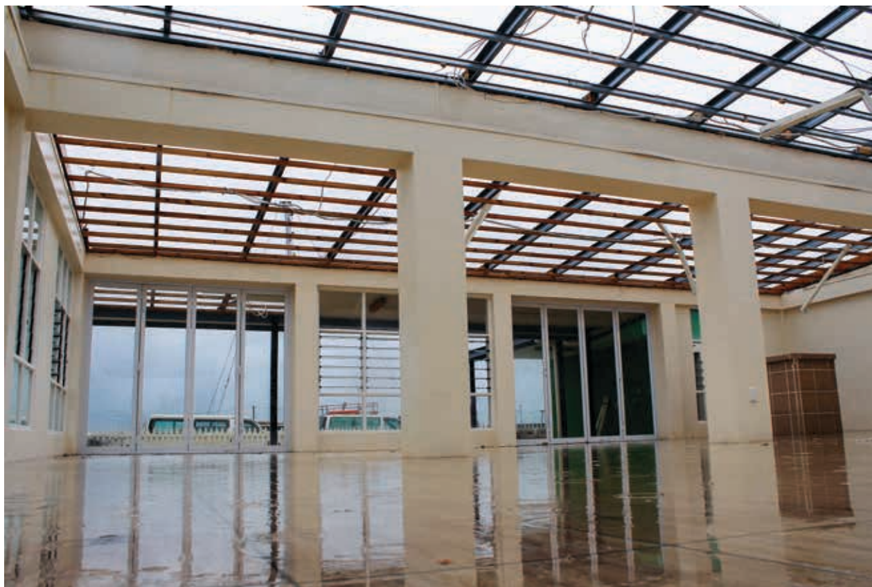
Photo: Malani Wolfgramm/World Bank. Damaged business, Tongatapu.
