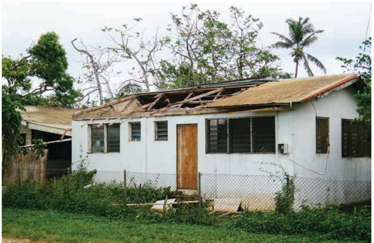
Photo: Malani Wolfgramm/World Bank. Damaged home in Longolongo, Tongatapu.
