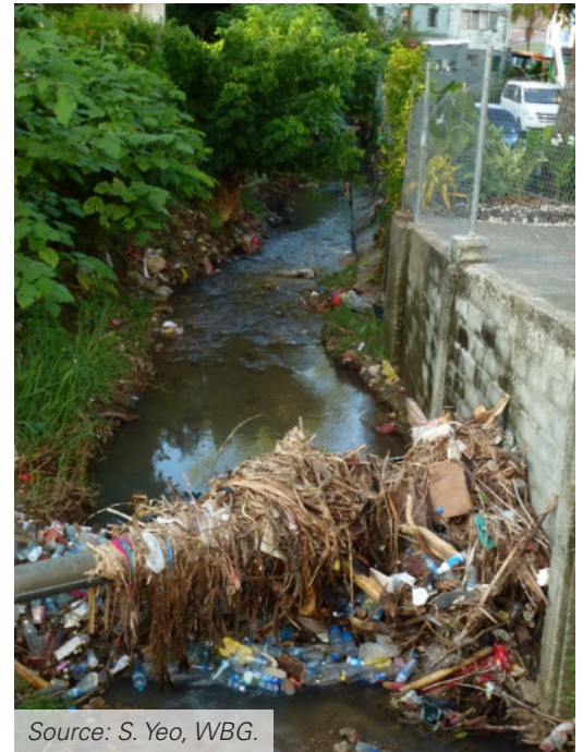
Figure 18. Solid waste limiting flow conveyance in a Honiara creek
