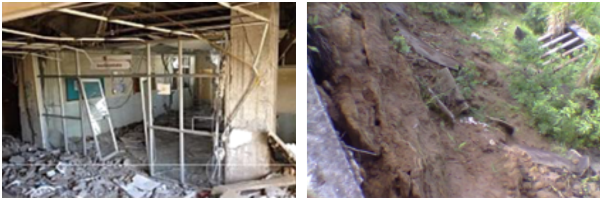
FIGURE 11: Seismically Damaged Critical Infrastructure
