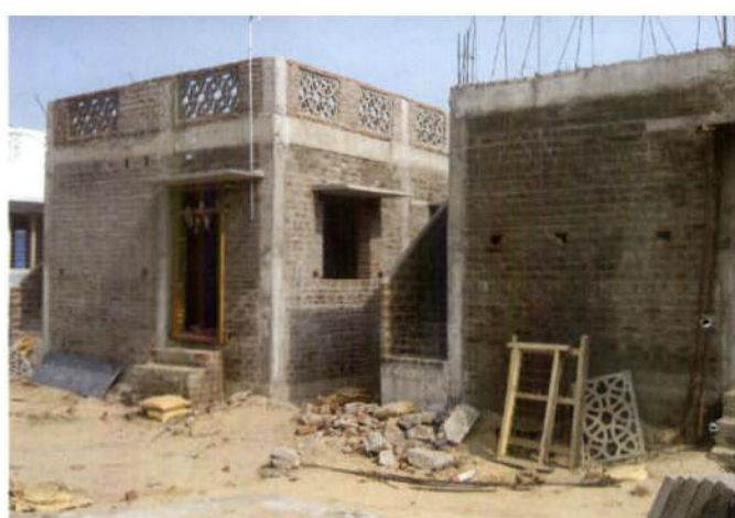
Houses under construction in Nagapattinam: Still many more have to be built
