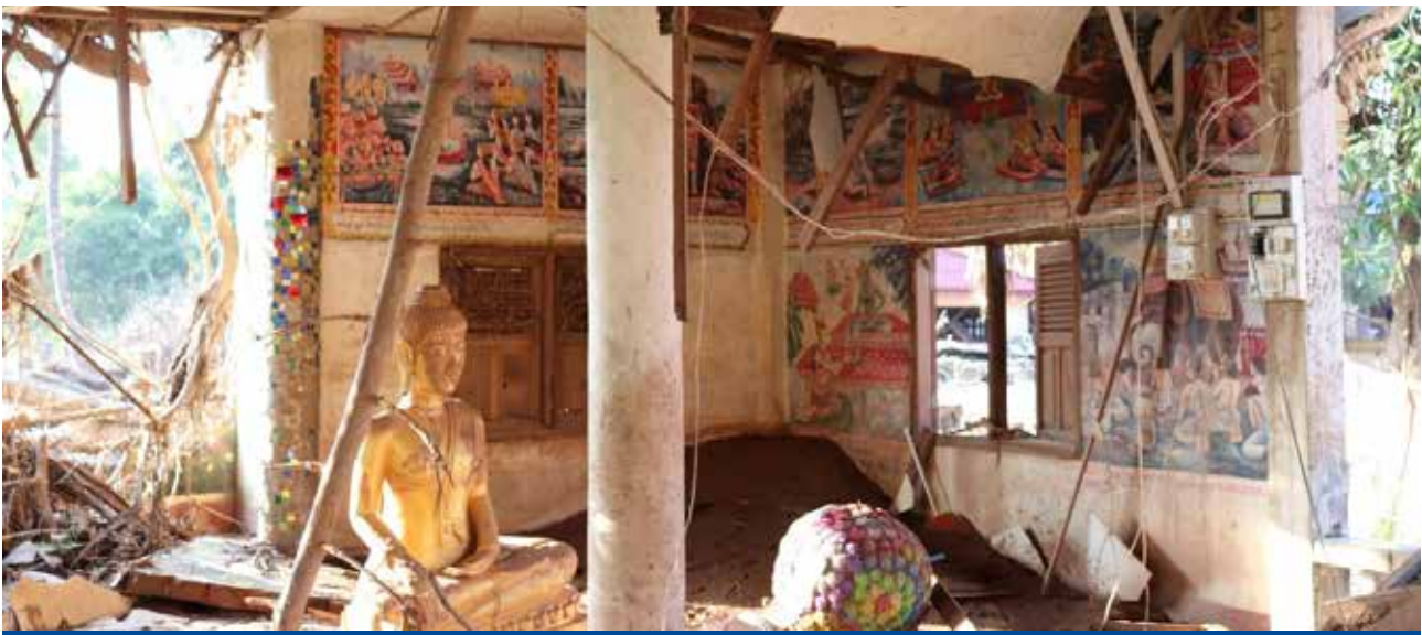
Damaged Temple at Vat Ban Mai, Sanamxay District, Attapeu Province.
