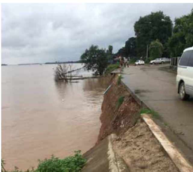
Damage to slope protection of Mekong mainstream, Thakek District, Khammuane Province.
