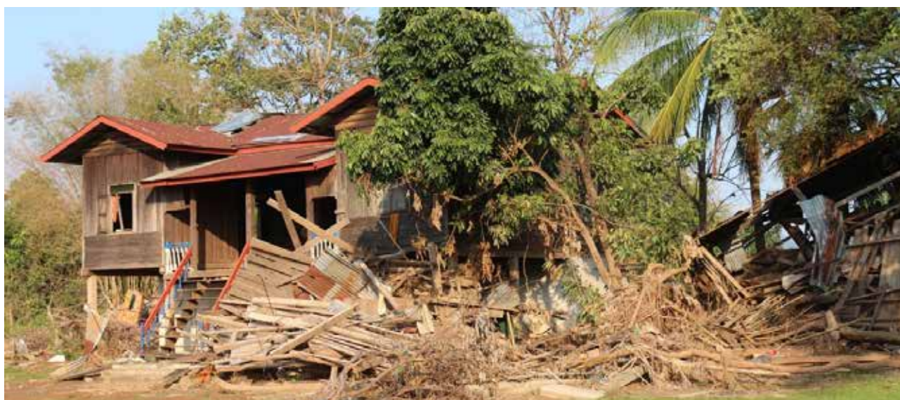
Damaged Kuti at Vat Ban Mai, Sanamxay District, Attapeu Province.
