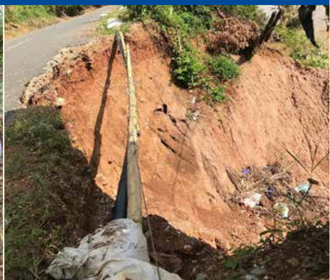
Damage on mainline distribution network of Nam Papa in Ngoy District, Luangprabang Province.
