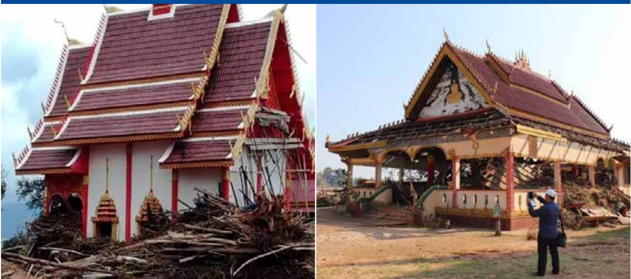
The damage at Vat Ban Hinlad, Sanamxay District, Attapeu Province.
