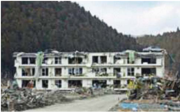
Figure 2.4 Reinforced concrete building withstood tsunami even though submerged (note car on roof)
