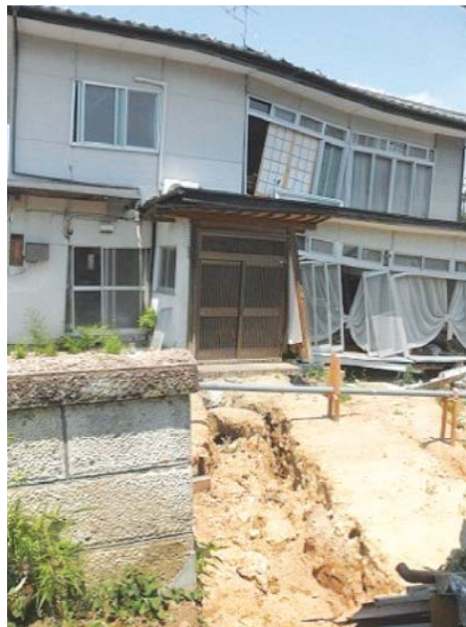
Figure 2.10 Houses damaged by failure of retaining walls
