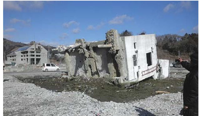
Figure 2.7 Overturned building of reinforced concrete with pile foundation
