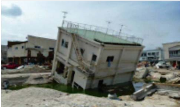
Figure 2.6 Reinforced concrete building scoured by the tsunami current
