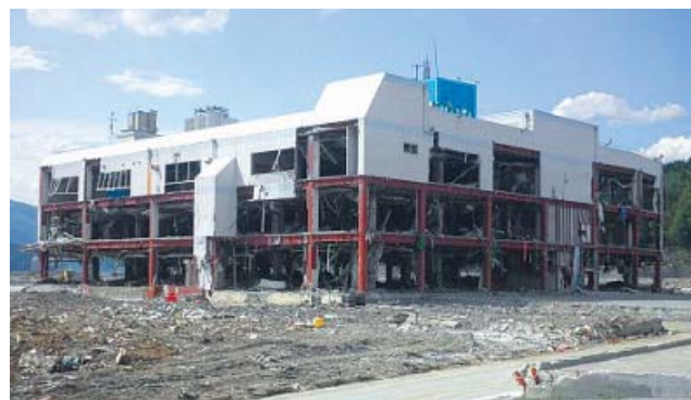
Figure 2.3 The tsunami destroyed the outer walls of steel structures
