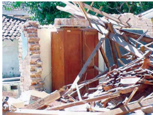
Figure 2.12 Collapsed school building in which furniture is still standing (Yogyakarta province, following Central Java Earthquake, 2006)
