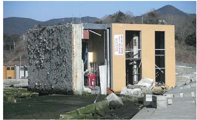
Figure 2.5 Reinforced concrete building damaged by buoyancy
