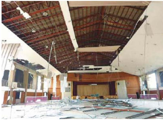
Figure 2.8 Fallen ceiling panels in school gymnasium
