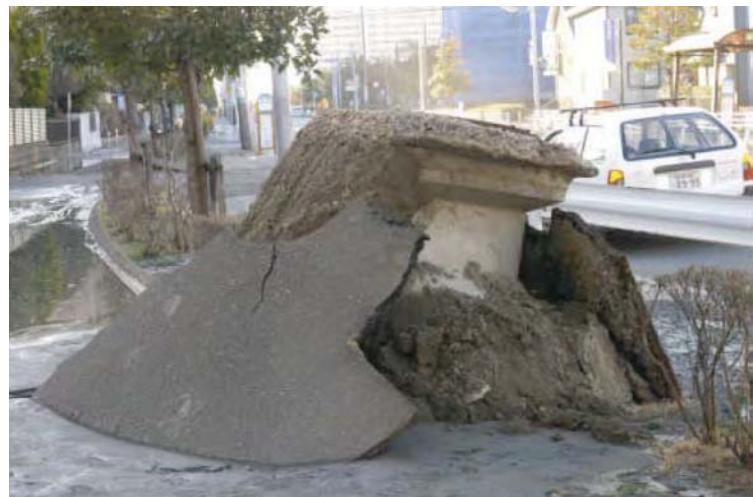
Figure 20.3 Manhole raised by liquefaction in Urayasu City
