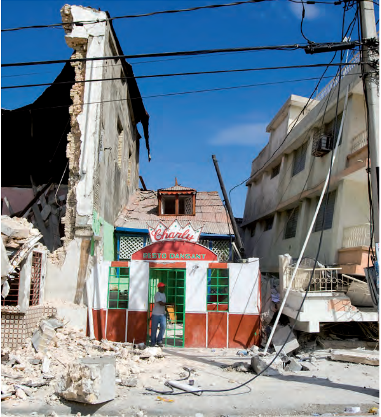
Port-au-Prince, Haiti, 2010: It is not the earthquakes that kill people, but the buildings collapsing on them.
