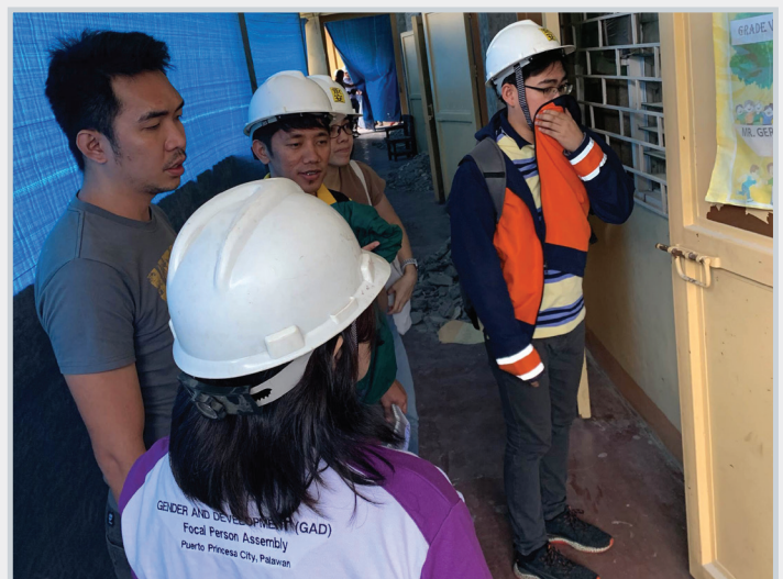
Above and facing page: Retrofitting of an elementary school in Metro Manila for seismic resilience funded by the Philippine government. Photos: World Bank.
