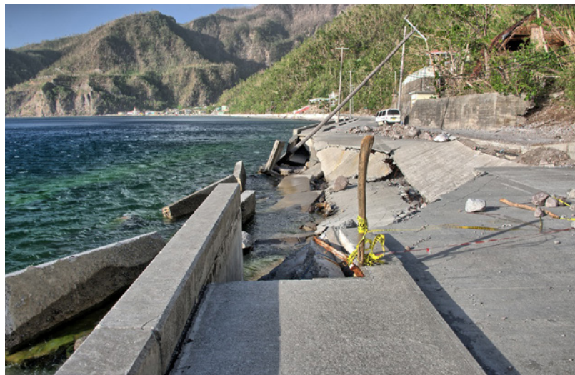
Figure C.16. Damaged Road Network in Dominica
