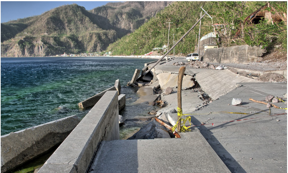
Figure 3.9. Damaged Road Network in Dominica following 2017 Hurricane Irma
