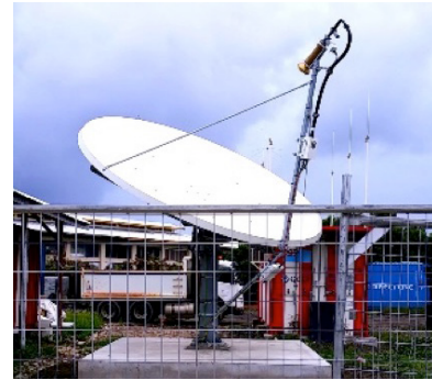
Figure C.34. VSAT Satellite Dish
