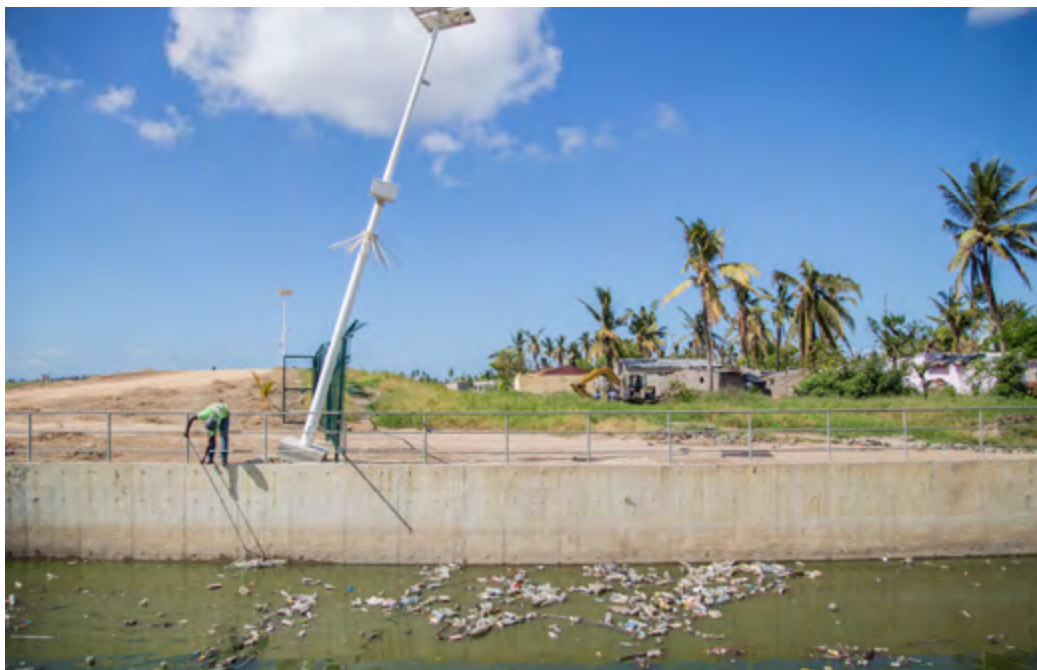
Municipal worker cleans canals that reduce the risk of flooding in Mozambique
