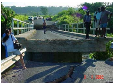
Figure 63: Failure of Teouma Bridge on the eastern access to Port Vila during 2002 earthquake
