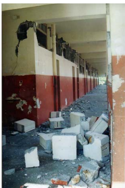
Figure 62: Structural failure of the lower floor of a 3-storey school classroom building during 2002 earthquake
