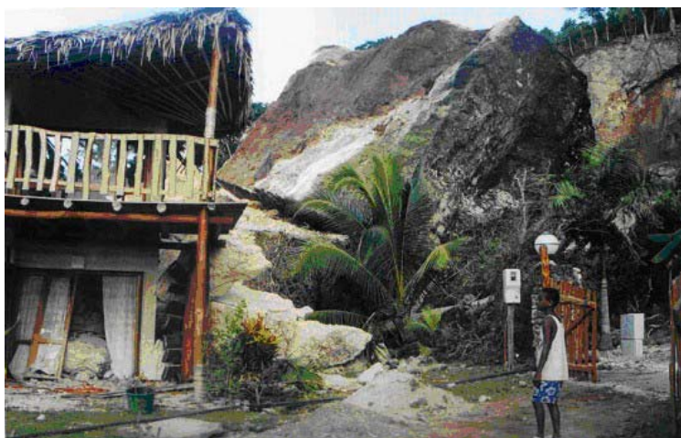
Figure 36: Toppling failure in limestone, destroying a coastal resort building
