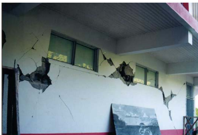
Figure 60: Structural damage to reinforced concrete Museum building during 2002 earthquake
