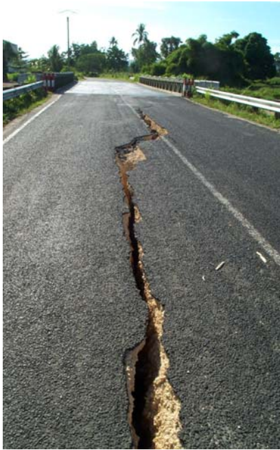
Figure 64: Failure of bridge approach embankment on western access to Port Vila during 2002 earthquake
