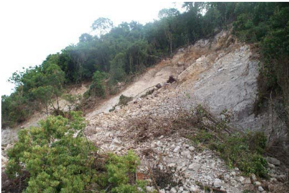
Figure 34: Slope failure in weak tuffaceous rock, blocking the main wharf access road - a limestone capping forms the cliff-line at the top of the slope
