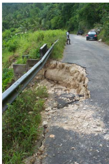
Figure 33: Roadway failure at the Klem’s Hill escarpment on the western access to Port Vila
