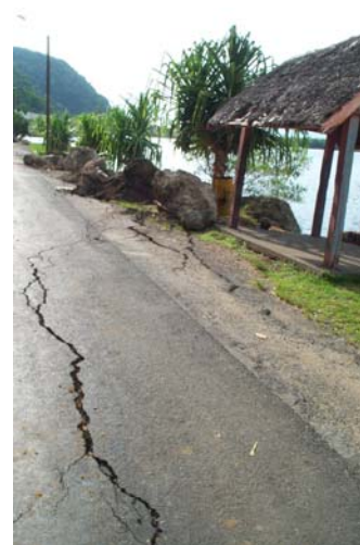
Figure 39: Fissuring and slumping of harbour-side roadway
