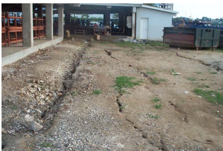
Figure 38: Settlement and fissuring of harbour-side fill at main city markets during 2002 earthquake
