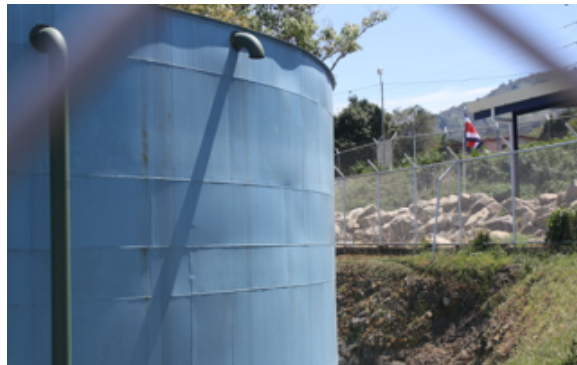
Figure 3 Detail of the metal walls of the Naranjal tank. The sheets forming the tank wall can be seen, as well as the welded seams, and the ripples which occur naturally in these kinds of welded joints.
