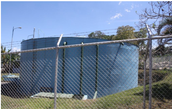
Figure 2 View from the outside of the metal Naranjal tank. At first glance it looks in good condition, with no visible areas of corrosion nor any loss of content.
