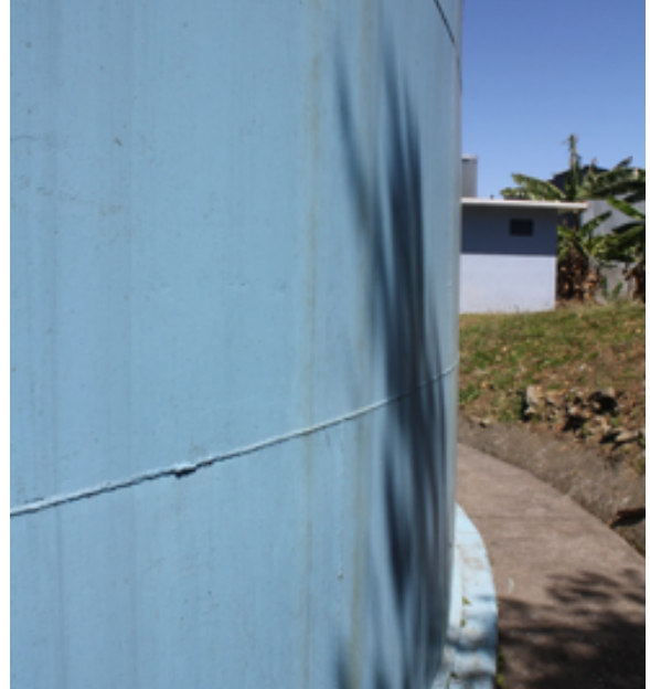
Figure 5 To the naked eye, the welded joints seem to be in good condition, although it is always possible to find some flaws in the welding work, which are, nonetheless, not serious.
