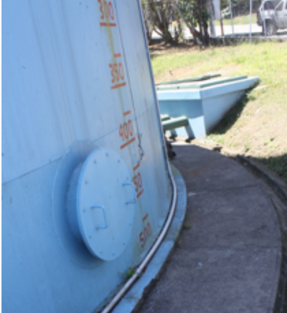
Figure 4 The Naranjal tank sits on a base of reinforced concrete, with no apparent anchor. At the time of inspection, the tank was almost full, and no loss of content could be seen at any point of the tank.
