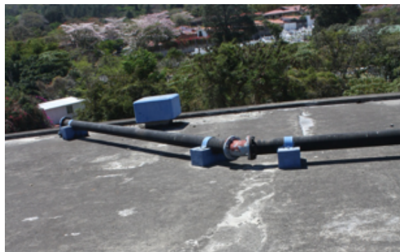
Figure 9 Picture of the Escazú Cemetery tank roof. Repairs are visible in well-defined areas.
