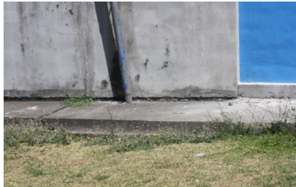
Figure 8 Evidence of compaction problems in the neighborhood of the Escazú Cemetery concrete tank
