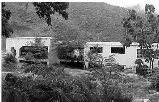
Bolivarian School after the 1999 torrential flow
