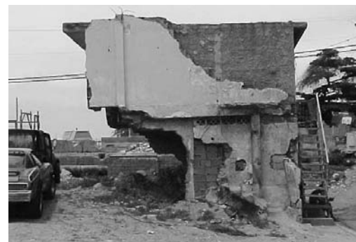
House affected by the 1999 torrential flow
