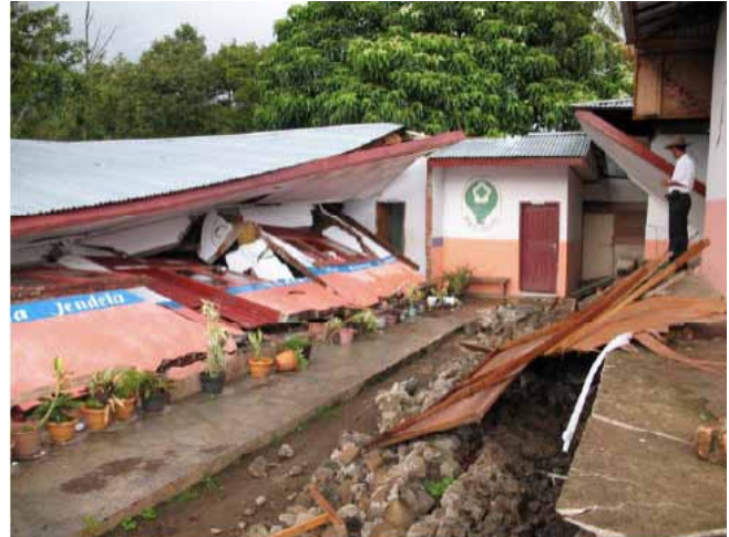
FIGURE 3. A collapsed school near the Sumatra Fault which caused the 2007 M6.3 West Sumatra earthquake. 700 school buildings were damaged in this moderate earthquake, 300 of which collapsed.
