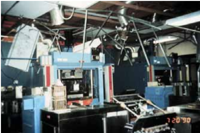
FIGURE 2. Damage to unprotected equipment and non-structural items in a clean room of an electronic components assembly plant, Baguio, Philippines, 1990 M7.7 earthquake. The building itself was not damaged significantly. The equipment damage caused a 3-month long business interruption and a major financial loss.
