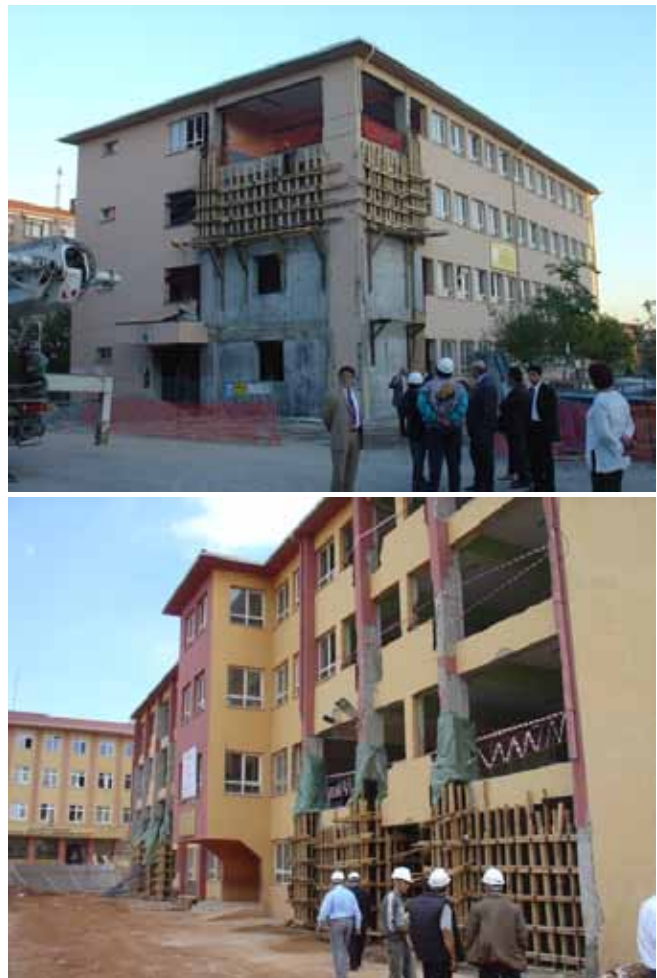
FIGURE 8. Three school buildings under construction in Istanbul. All are completed today. Additional reinforced concrete walls are being added to strengthen the buildings.
