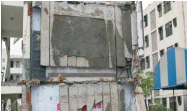
FIGURE 5. Partial view of the interior of three vertically stacked school rooms in a collapsed middle school in Dujiangyan; 2009 M7.9 Sichuan, China earthquake.
