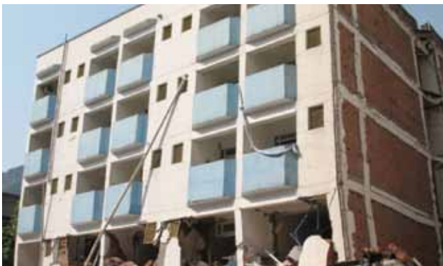
FIGURE 6. Collapsed ground floor of a hospital building in Mianzhu, 2009 M7.9 Sichuan, China earthquake.
