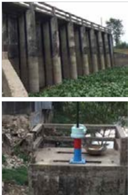
FIGURE 4.3. POORLY MAINTAINED REGULATORS IN DHAKA WEST
